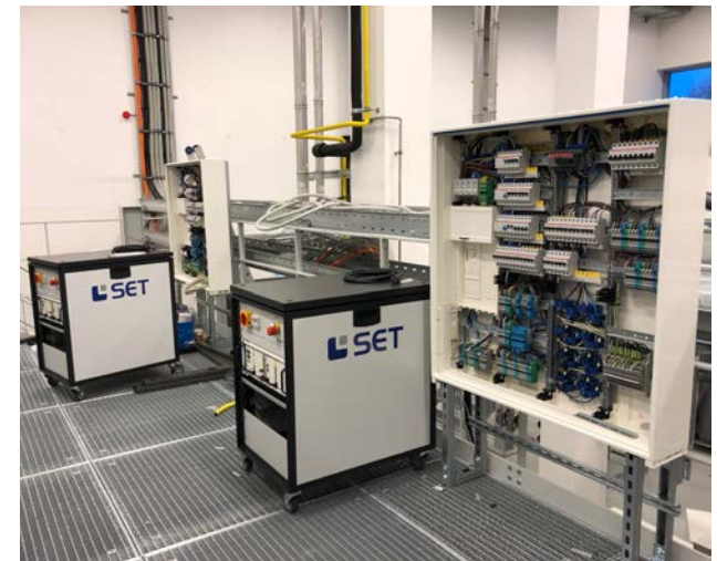
Power Grid Control
