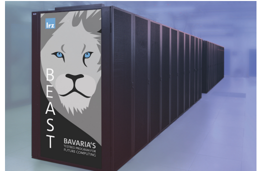
BEAST Bavarian Energy, Architecture, and Software Testbed @ LRZ
